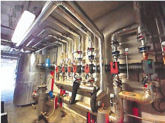
Process chaudière Bois
