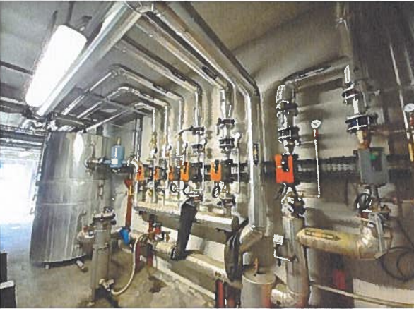
Process chaudière Bois
