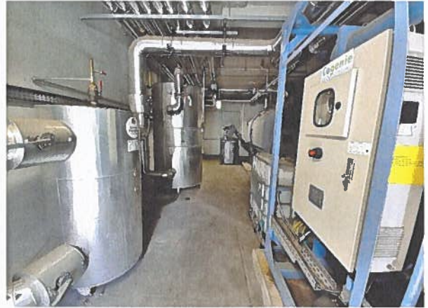
Process chaudière Bois
